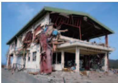
Disaster damaged former Kirikiri Nursery School building
