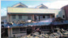
Midori Kindergarten after the earthquake. The school was in a relatively new building that was constructed only about five years ago. (Photograph provided by Midori Kindergarten)
