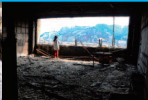
A classroom on the second floor of Otsuchi Primary School was burnt black after the tsunami and fires.— Photo by Kenichi Shindo on 31 March 2011 at Otsuchi town, Iwate Prefecture.
